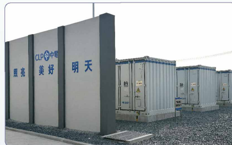
The battery energy storage system at Jiangsu Yixing I Power Station
